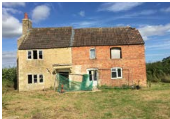
PRE-BUILD The original buildings on the site when the plot was bought at auction were a pair of derelict farm cottages.
