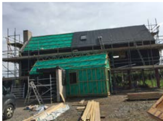
ROOF AND WALLS Weathertight is achieved. A utility and pantry sit at the front of the house in a small entry wing.
