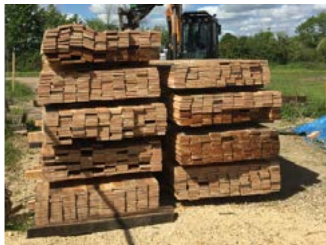
MATERIALS Larch hardwood timber was selected by Antony and Jenni for the shou sugi ban charred timber cladding.
