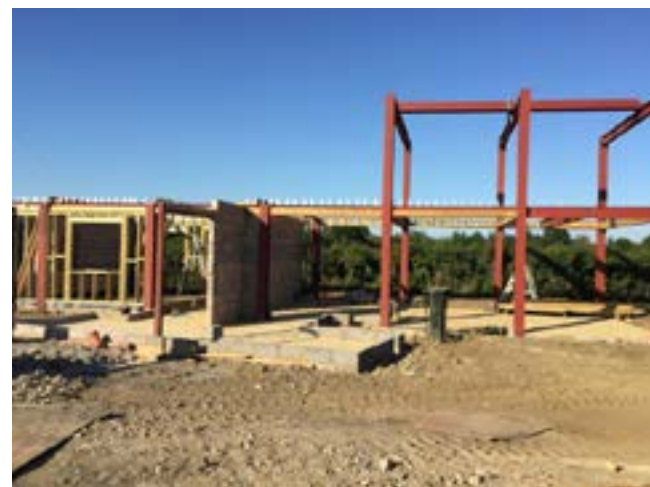
STEEL FRAME Erected in just one day, the property's steel frame underlays the charred timber cladding.
